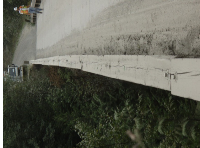
Figure 12: Span 1 looking toward the right abutment (North Bend). Kink in downstream curb at Pier #1; due to failure of 3 of 4 Span 1 anchor bolts at Pier #1.
