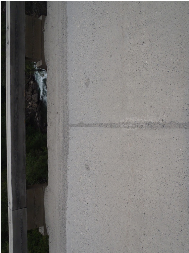
Figure 13: Typical condition of grouted deck joint.
