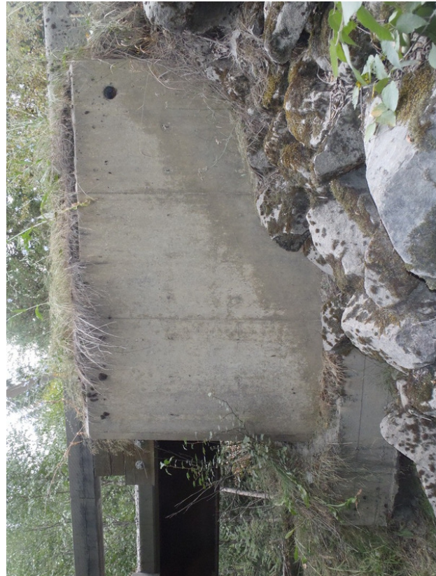
Figure 24: Right end upstream wingwall (upper) - note loss of fill below footing.
