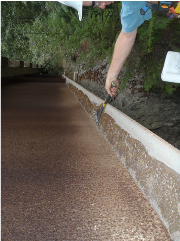
Figure 17: Typical debris accumulation along bottom flange - Span 2 downstream shown.
