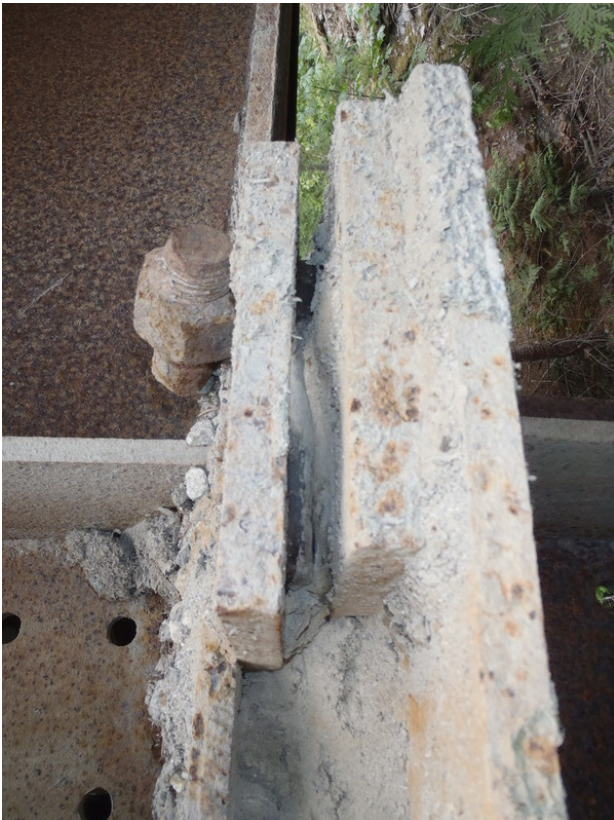
Figure 33: Pier 1 span 1 downstream bearing - Note failed anchor bolt.
