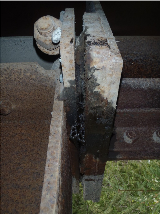
Figure 34: Pier 1 Span 1 bearing - Note bearing squeezed out.
