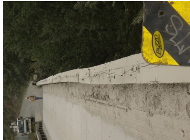
Figure 11: Span 1 looking toward the right abutment (North Bend). Kink in upstream curb at Pier #1; due to failure of 3 of 4 Span 1 anchor bolts at Pier #1.
