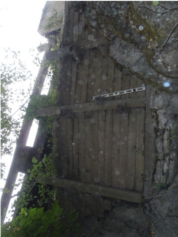
Figure 25: Right end upstream wingwall (lower) - note condition of tiebacks.
