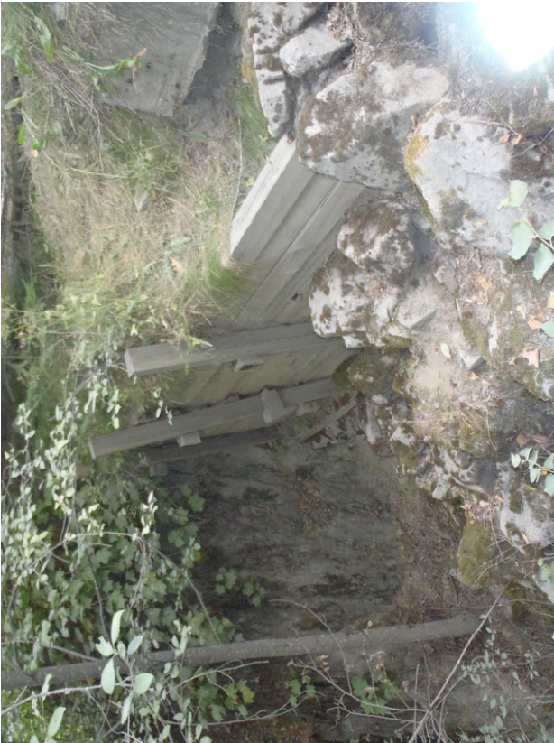
Figure 26: Right end upstream wingwall (lower) - note rotation of wall.
