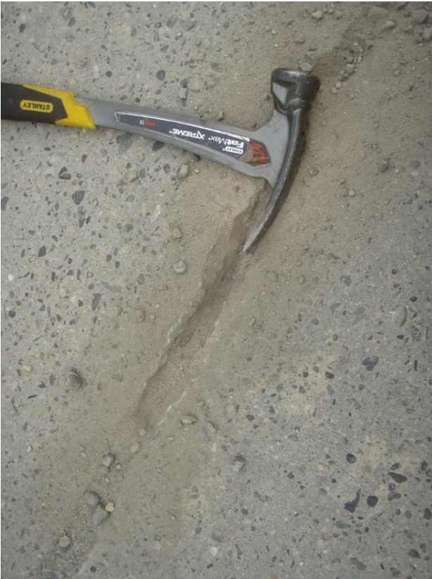
Figure 14: Typical deterioration of grouted deck joint.
